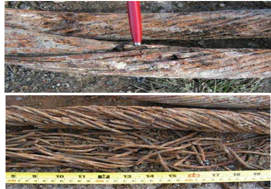
Corroded and fractured outer A gal. wires of 6-strand catenary line from Kumul SPM recovered after 4.5 years in tropical water.
